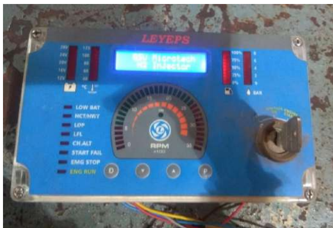
FIGURE 4. ECU to Control MEA Injection
