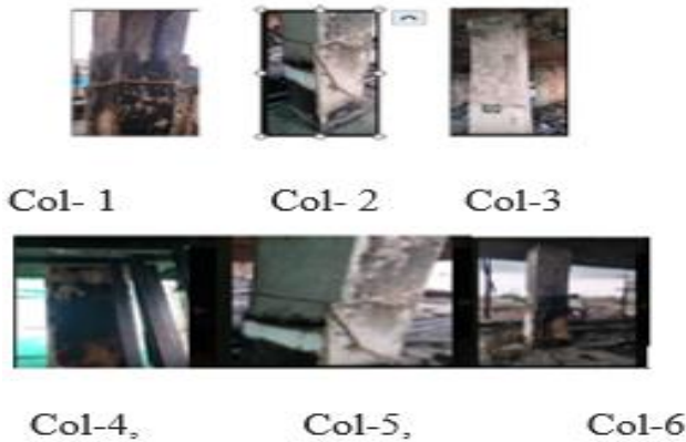
Figure 7 Condition of The Column on Floor 4
