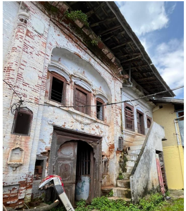
Figure 5 Abandoned Haveli, Pragpur
